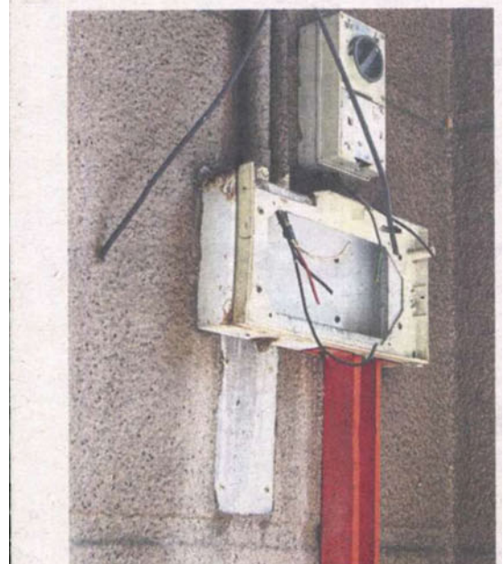
Exposed and broken cables can be seen in Taman Seratus, Klang.
