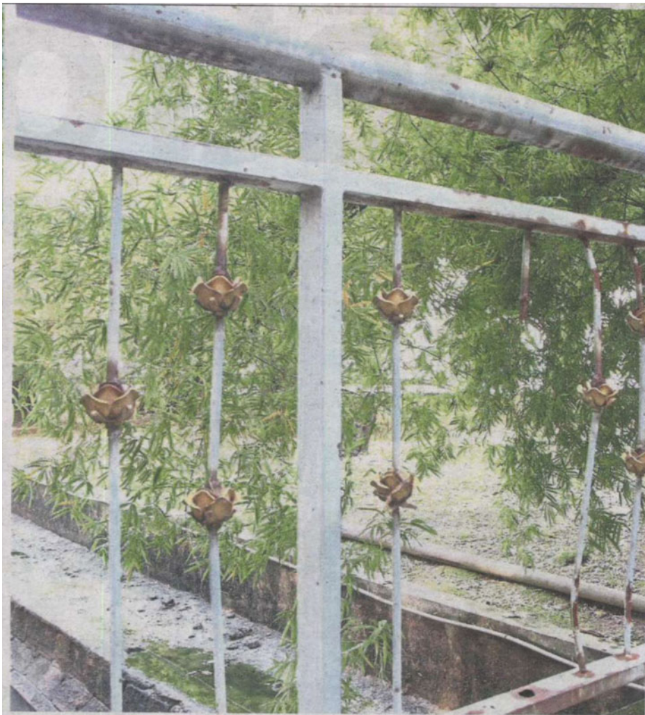
Missing railings at Taman Seratus poses as a danger to the children playing there. — Photos: SAMUEL ONG/The Star
